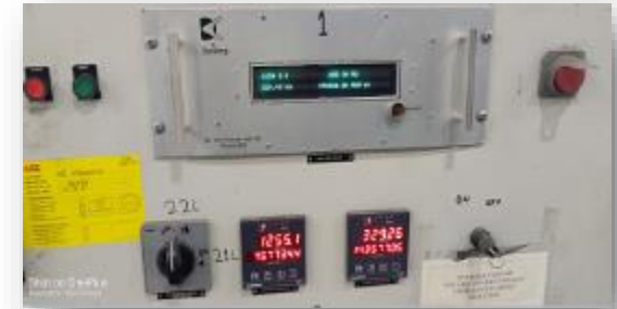
Integrated Energy Meters
